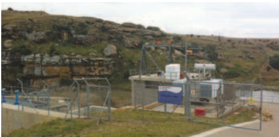
Bethlehem Hydro's Sol Plaatje power station.
